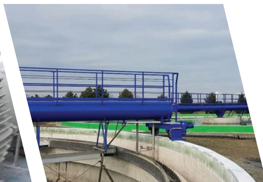
Čakovec Wastewater Treatment Plant
